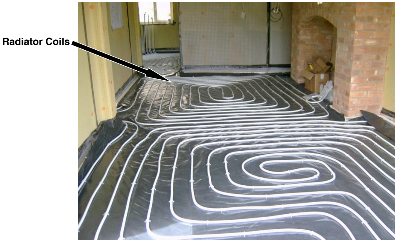
Figure 9 – Hollow coils located beneath the floor [25]
